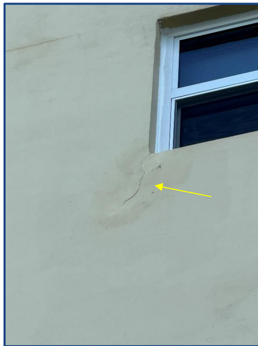
Photograph No. 50: Wall cracking observed at X05/X06 riser.
