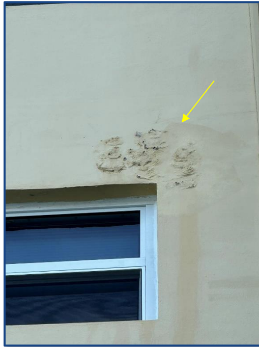
Photograph No. 51: Wall cracking observed at X05/X06 riser.
