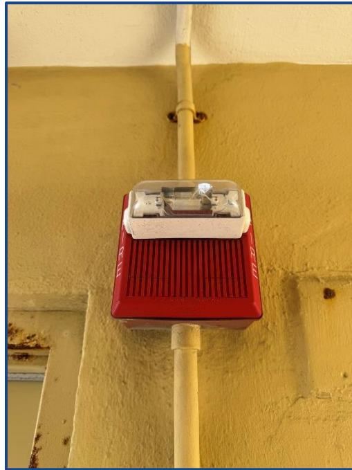
Photograph No. 17: Building Typical Fire Siren and Fire Emergency Light
