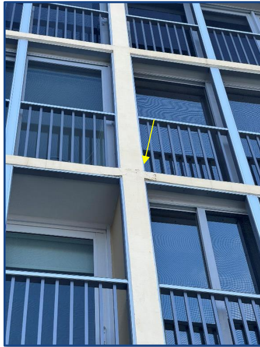
Photograph No. 37: Edge cracking observed at X01/X02 riser.
