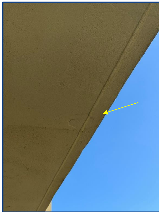
Photograph No. 26: Overhead cracking observed near unit 604.
