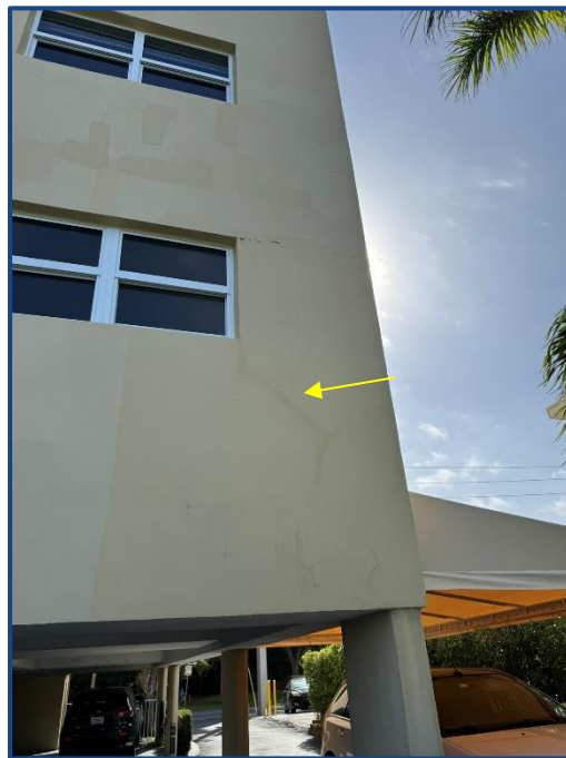
Photograph No. 40: Wall cracking observed at X01 window riser.
