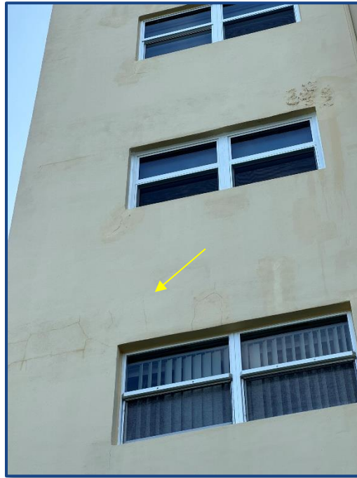
Photograph No. 49: Wall cracking observed at X05/X06 riser.
