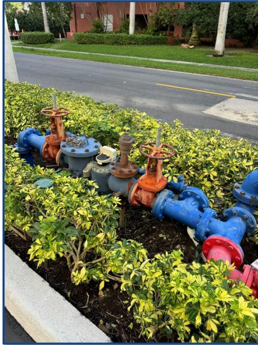
Photograph No. 21: Building Backflow Preventer & Double Detector Check Valve
