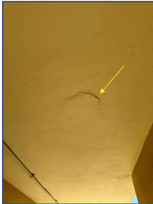
Photograph No. 24: Overhead spalling observed near unit 701.
