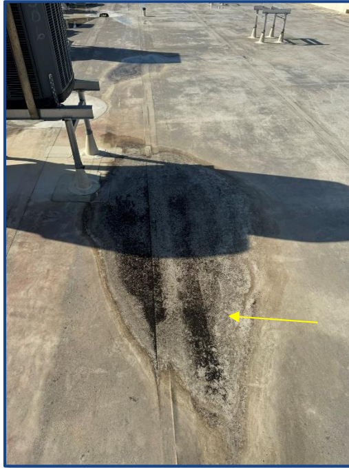
Photograph No. 69: Debris buildup observed from water accumulation at building roof.
