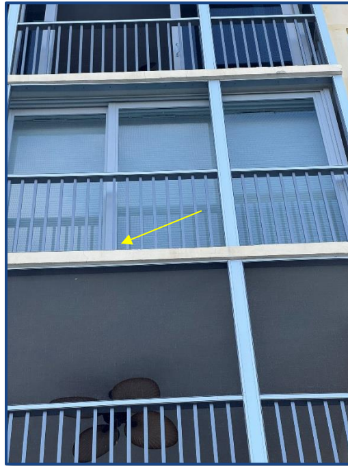
Photograph No. 45: Edge cracking observed at X03/X04 riser.
