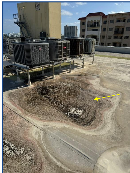
Photograph No. 66: Debris buildup observed from water accumulation at building roof.
