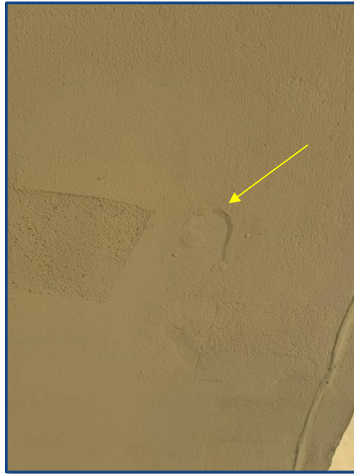
Photograph No. 25: Overhead cracking observed near unit 705.
