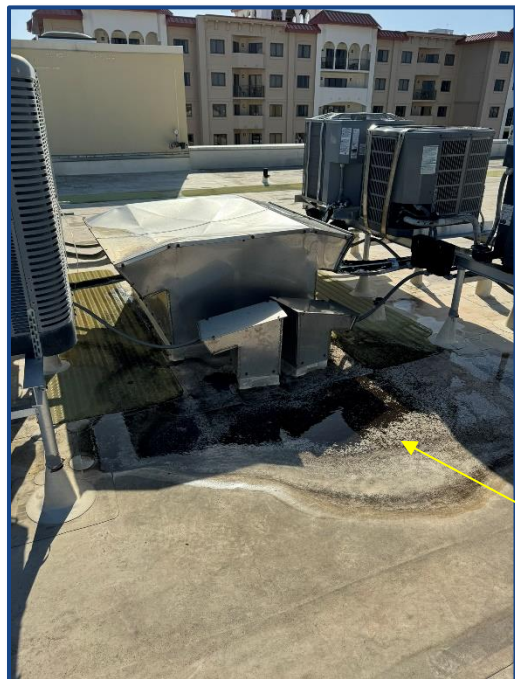
Photograph No. 68: Debris buildup observed from water accumulation at building roof.
