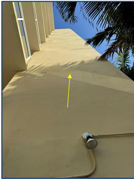
Photograph No. 32: Wall cracking observed at South stairs 2 nd floor.
