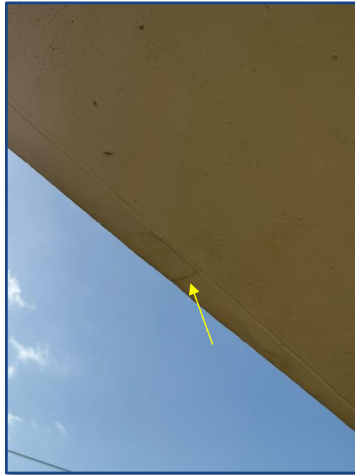
Photograph No. 29: Overhead cracking observed near unit 401.
