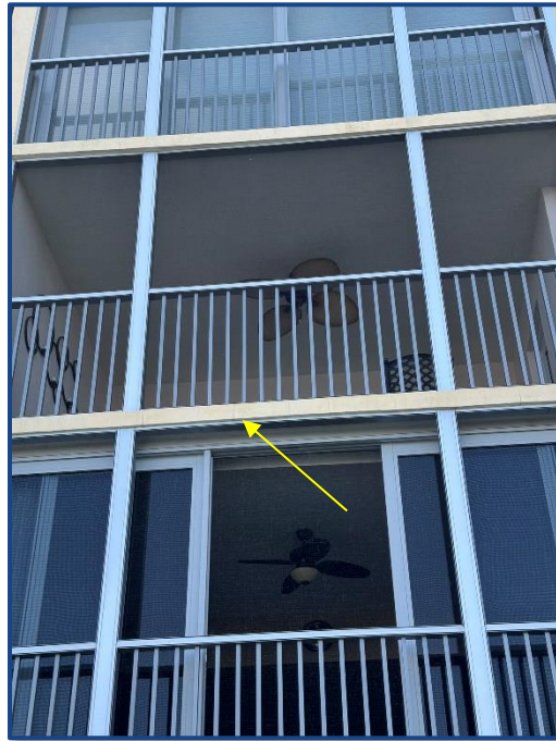
Photograph No. 43: Edge cracking observed at X03/X04 riser.
