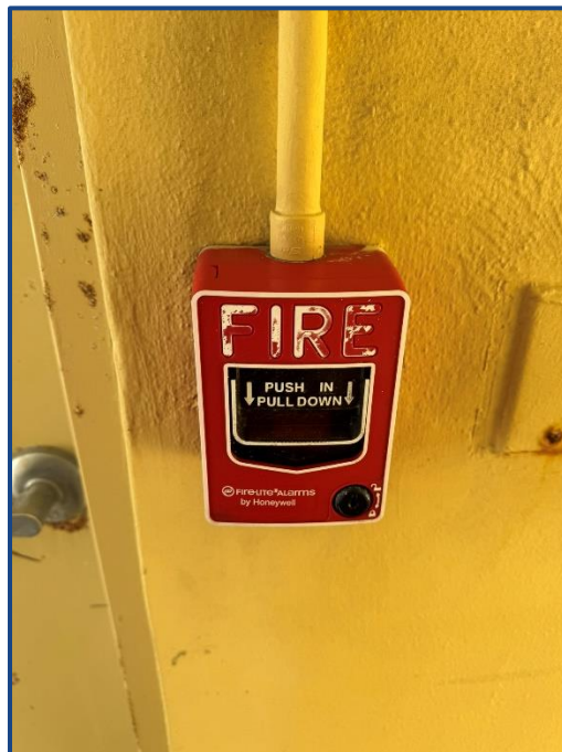
Photograph No. 16: Building Typical Fire Alarm Pull Station
