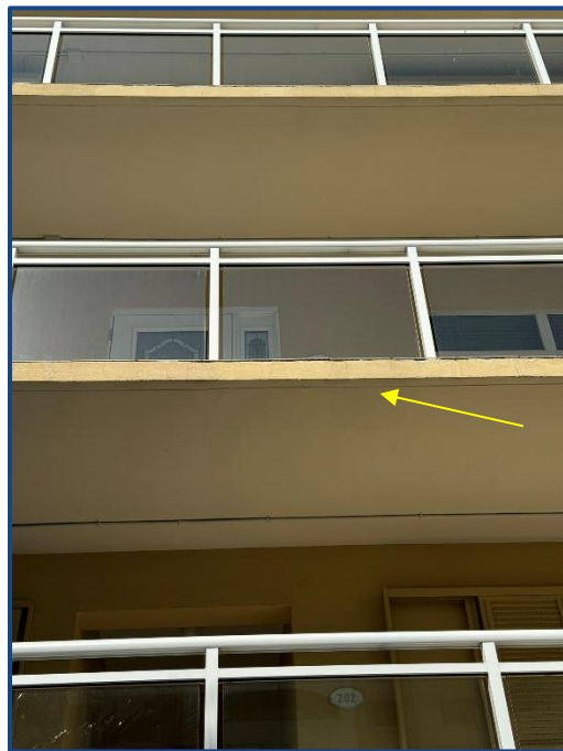
Photograph No. 60: Edge cracking observed near riser X02 catwalk side.
