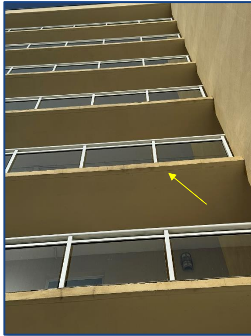
Photograph No. 55: Edge cracking observed near riser X05 catwalk side.
