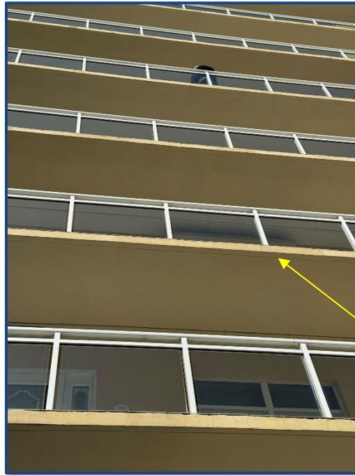
Photograph No. 61: Edge cracking observed near riser X02 catwalk side.
