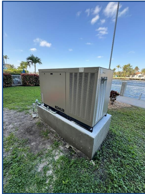
Photograph No. 15: Building Generator
