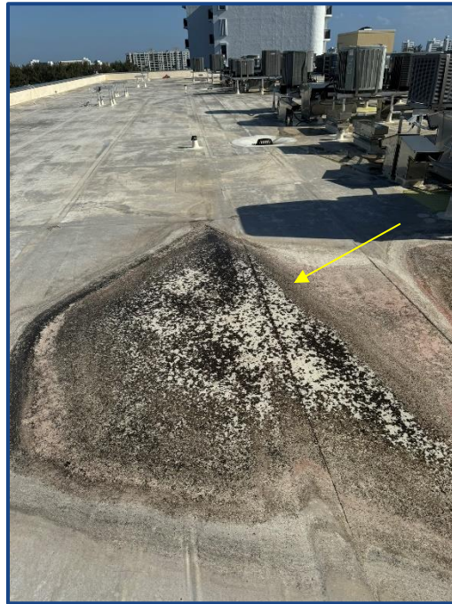
Photograph No. 67: Debris buildup observed from water accumulation at building roof.
