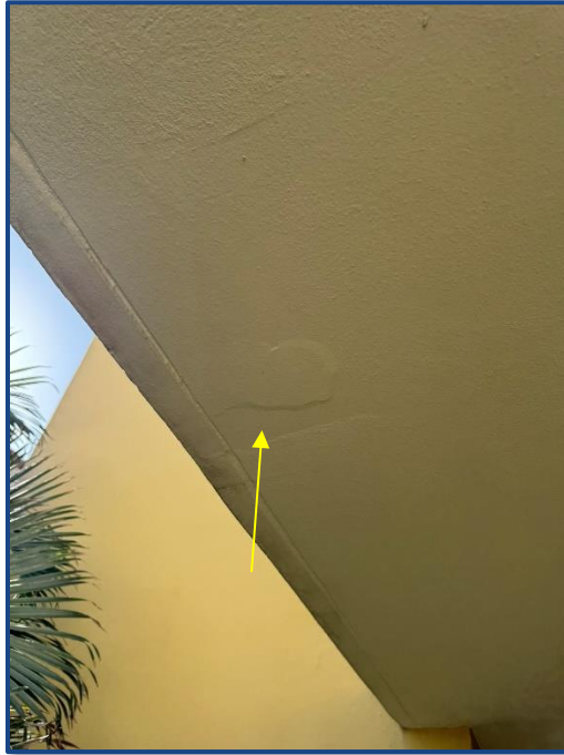
Photograph No. 31: Overhead spalling observed near unit 202.
