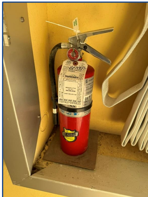
Photograph No. 20: Building Typical Fire Extinguisher
