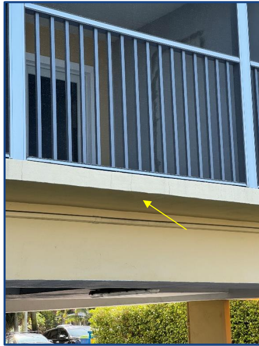
Photograph No. 35: Edge cracking observed at X01/X02 riser.
