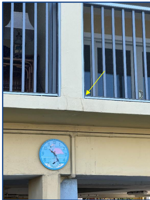
Photograph No. 34: Edge cracking observed at X01/X02 riser.
