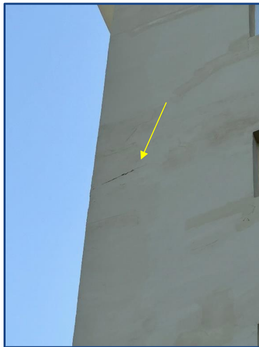
Photograph No. 52: Wall cracking observed at X05/X06 riser.
