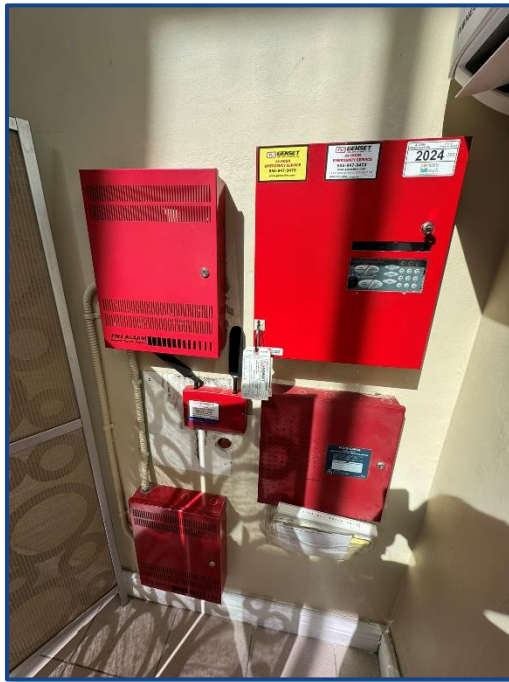
Photograph No. 22: Building Fire Alarm Panel
