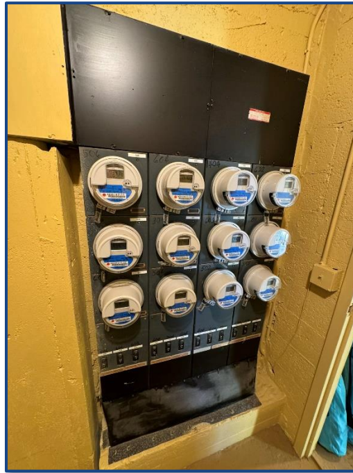
Photograph No. 13: Building 5 th Floor Electrical Room
