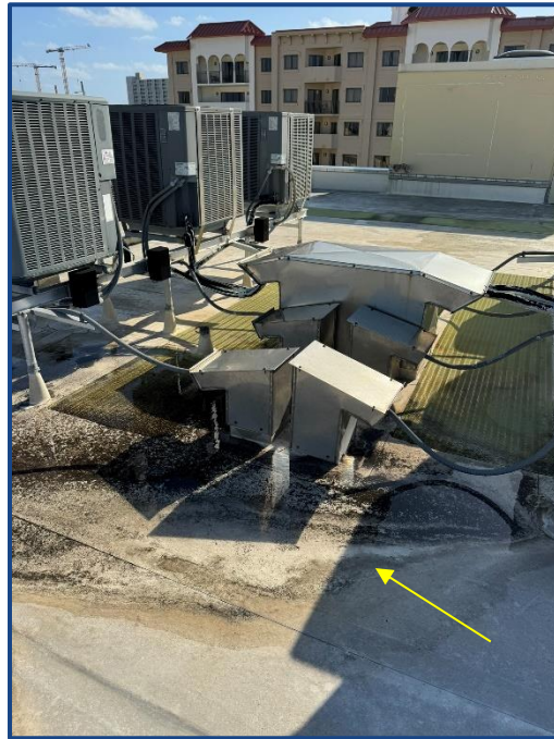
Photograph No. 65: Debris buildup observed from water accumulation at building roof.
