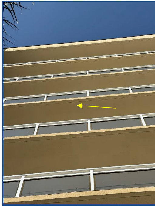
Photograph No. 59: Edge cracking observed near riser X05 catwalk side.
