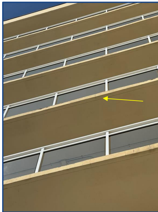
Photograph No. 56: Edge cracking observed near riser X05 catwalk side.
