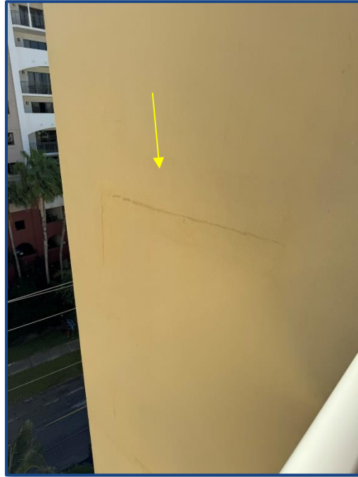
Photograph No. 23: Wall cracking observed at South stair tower 7 th floor.
