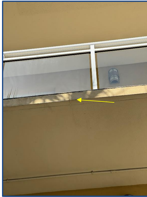
Photograph No. 57: Edge cracking observed near riser X05 catwalk side.
