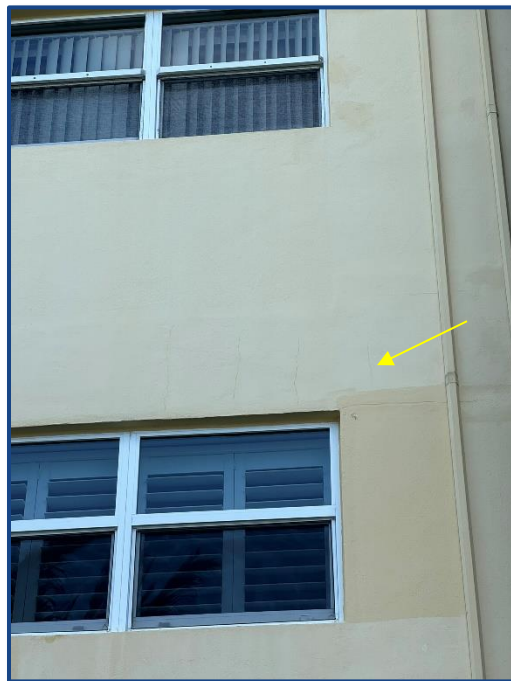
Photograph No. 48: Wall cracking observed at X05/X06 riser.
