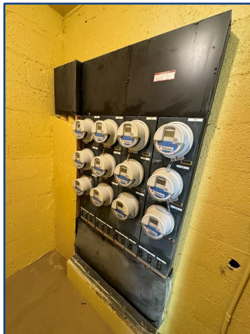
Photograph No. 12: Building 7 th Floor Electrical Room
