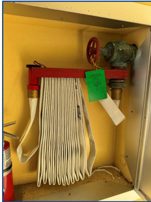
Photograph No. 19: Building Typical Fire Hose Station
