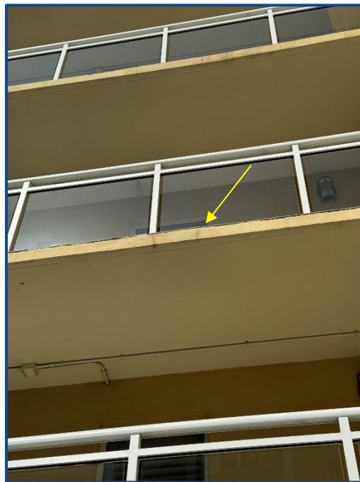
Photograph No. 54: Edge cracking observed near riser X05 catwalk side.
