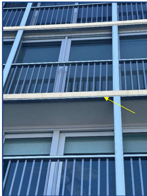
Photograph No. 38: Edge cracking observed at X01/X02 riser.
