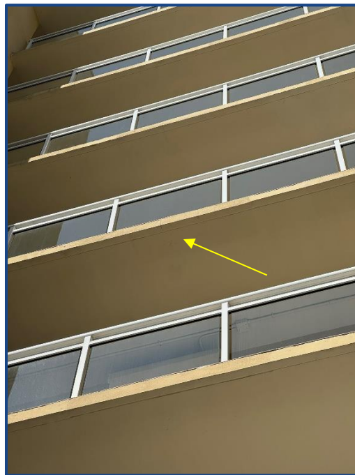
Photograph No. 62: Edge cracking observed near riser X02 catwalk side.
