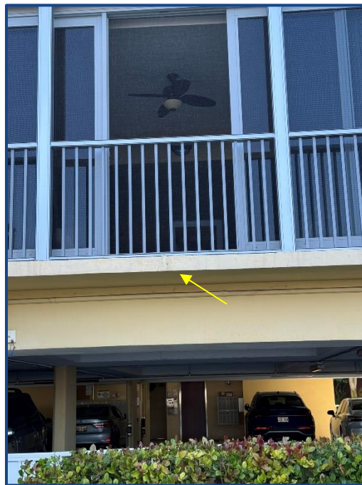
Photograph No. 42: Edge cracking observed at X03/X04 riser.
