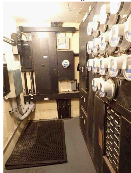
electrical meter room
