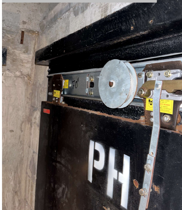
Hoistway door track and hardware needs cleaning and lubrication.
