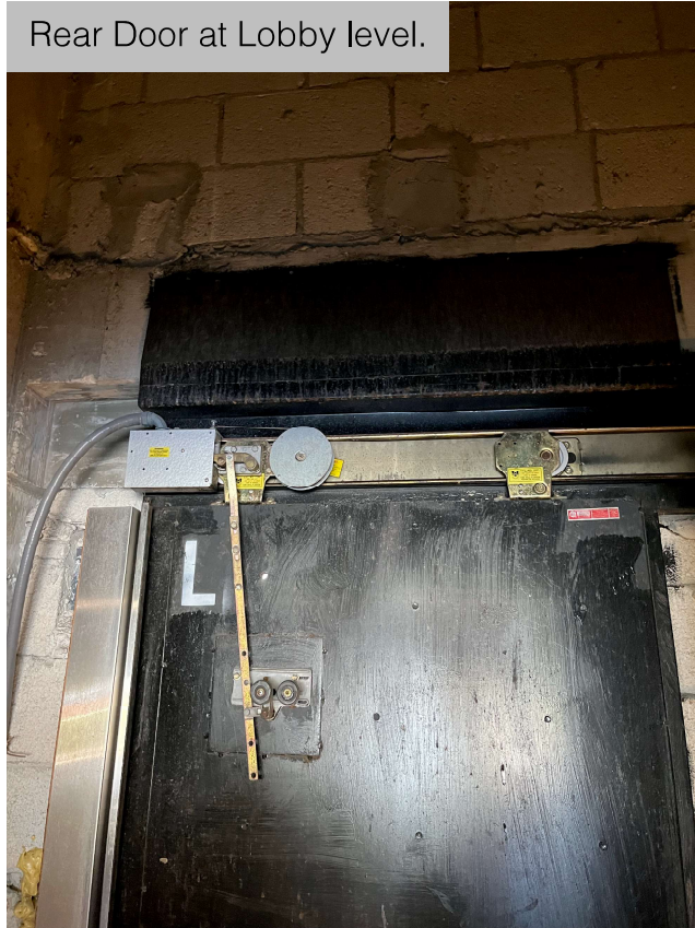
Pit area - Needs cleaning. Excessive wires plugged into outlet does not meet code.
