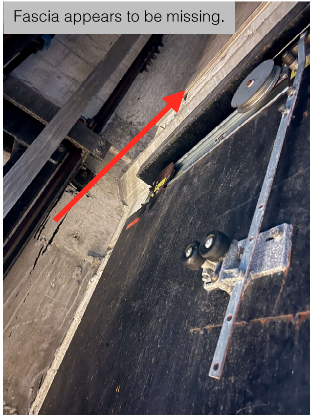
Typical rusty door track. Also, exposed wires behind the jamb does not meet code.
