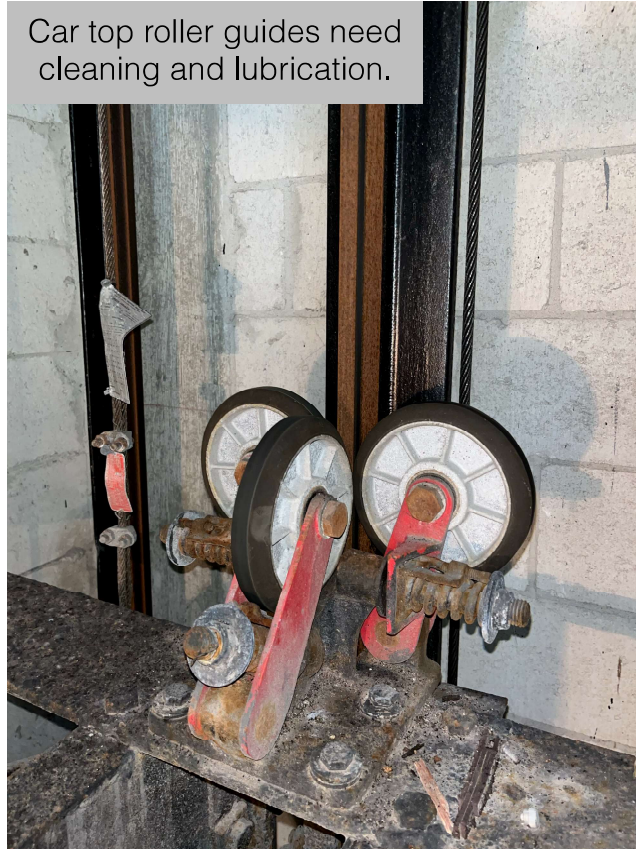
Selector tape is stainless steel and in good condition.
