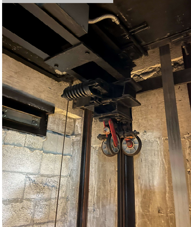
Car safeties appear to be in good condition.
