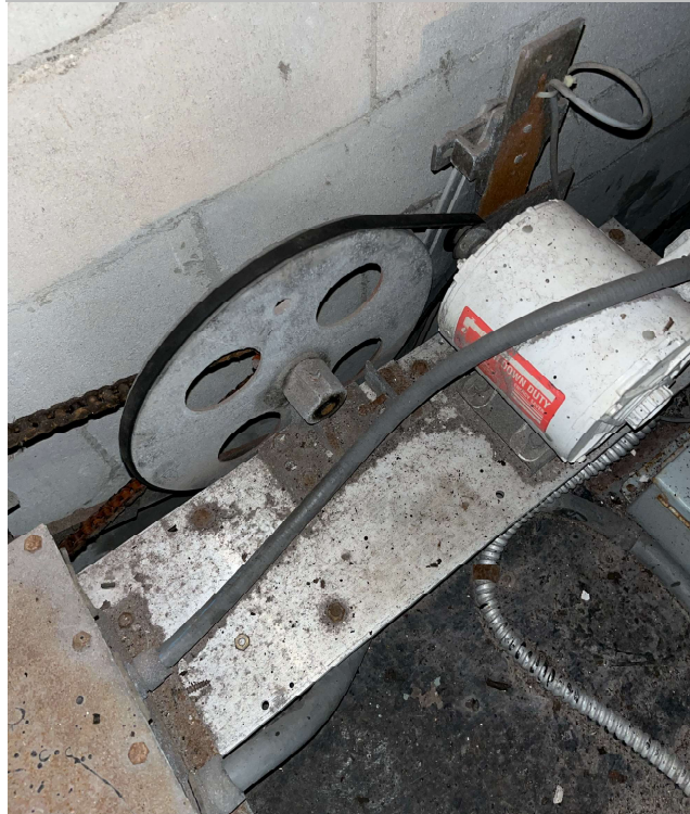
This is a GAL water resistant door operator. It needs cleaning and lubrication.
